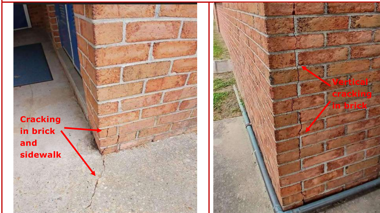
Pictures illustrating minor cracking observed near building corners.
